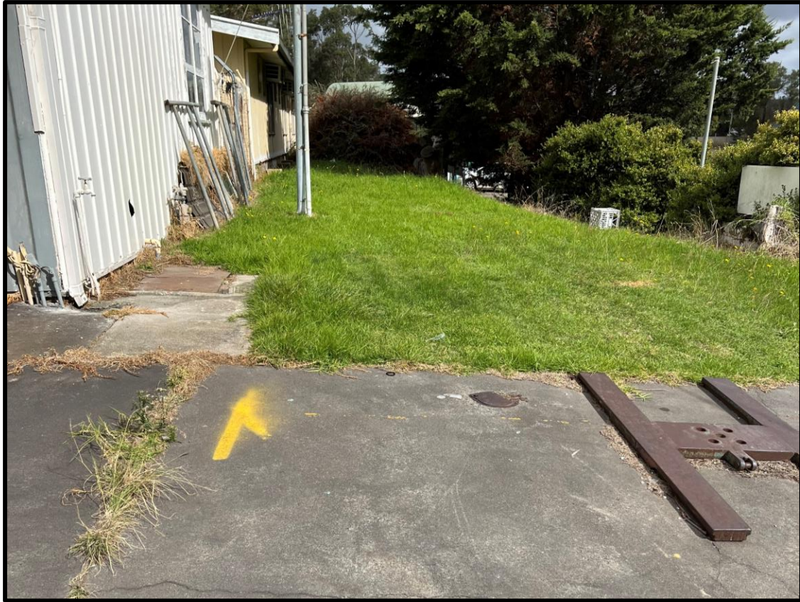
Figure 11. Suspect waste oil tank within south-western portion of the site.
