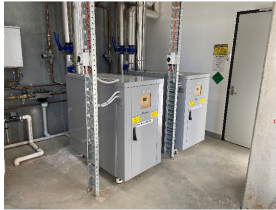
Indoor Plant Room – Boilers
