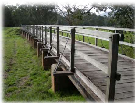
Re-constructed railway bridges, complete with decking and handrails, on the Lilydale Warburton Rail Trail in Victoria. Bridges were re-built by the Country Fire Authority, which used the contract fee to acquire a new fire tender.
