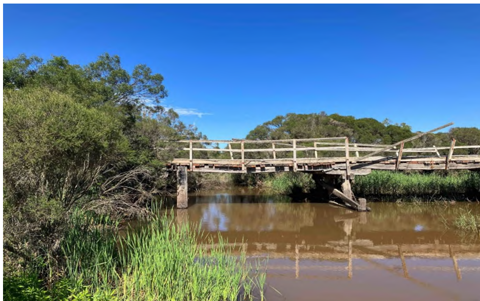
Mayfield Road Bridge is currently closed to the public. Traffic diversions are in place
