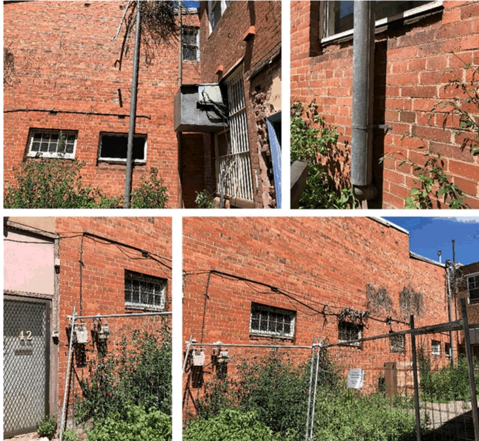
Figure 4 – Windows on adjoining property at 201 Auburn St
