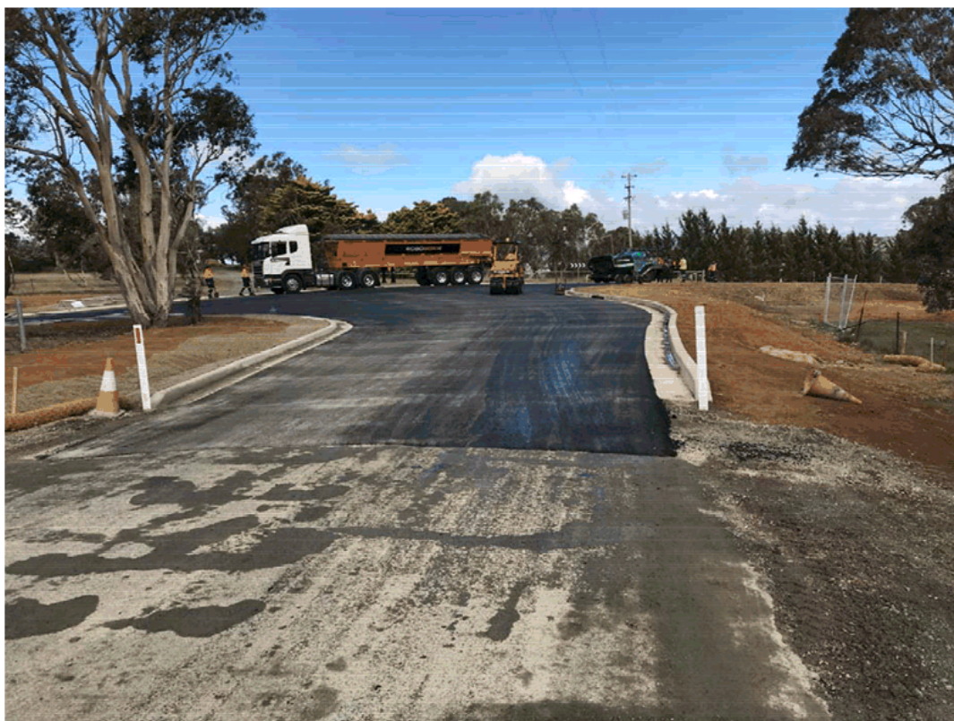
Laying of asphalt at the intersection of Mary Street and Ridge Street
