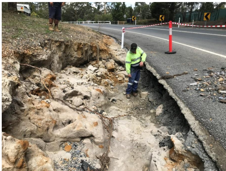
Highlands Way - depth of scour Viaduct
