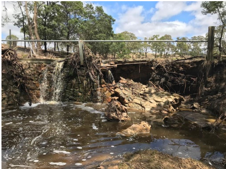
ch 5.5km Forest Siding Road damaged causeway 3
