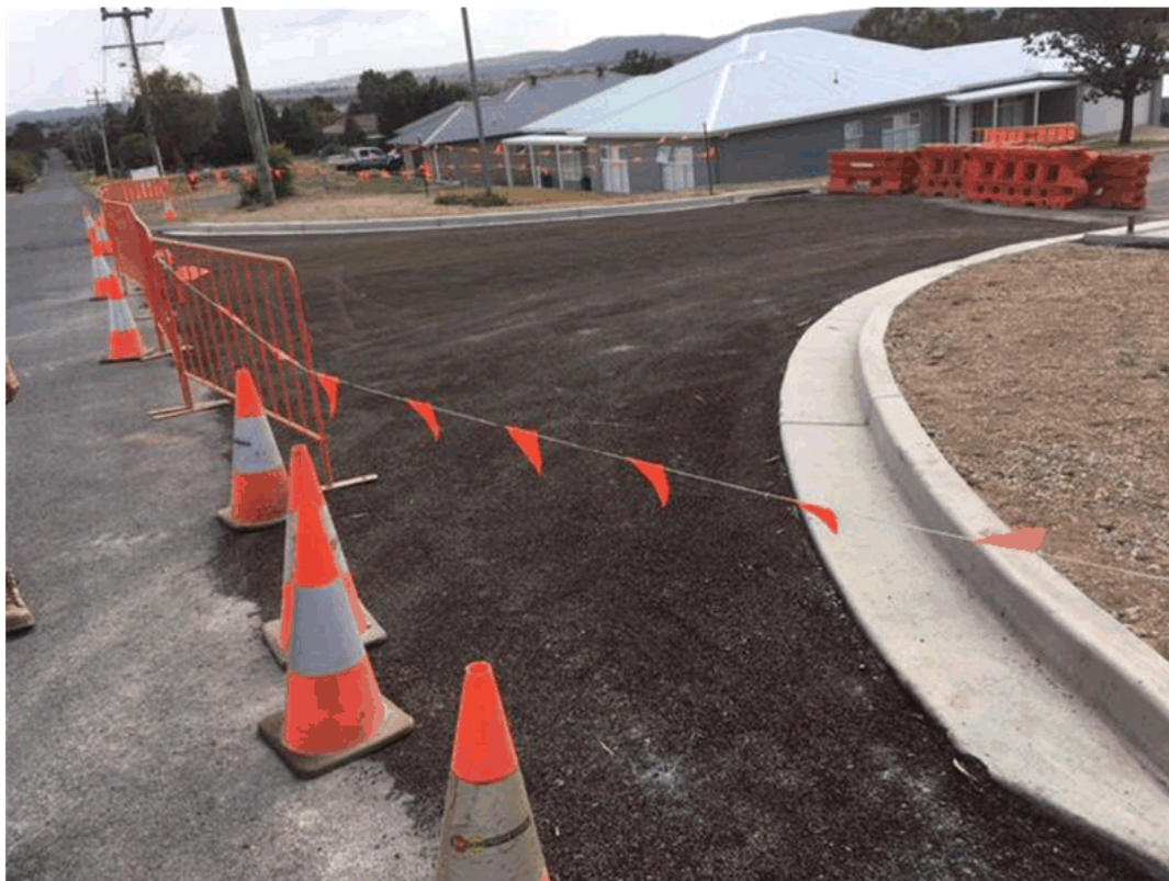
Sanctuary Drive / River Street Intersection - New kerb, gravel and prime seal ready for asphalt
